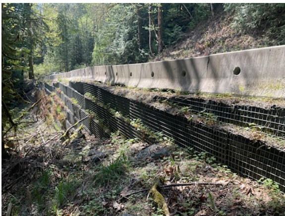
Geotextile and wwm in good shape. Minor bulging but not severe. Bulging exists where wwm not tied back because cut.
